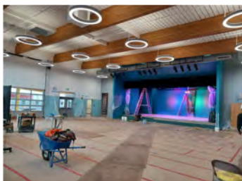
Cafeteria Stage Lighting
